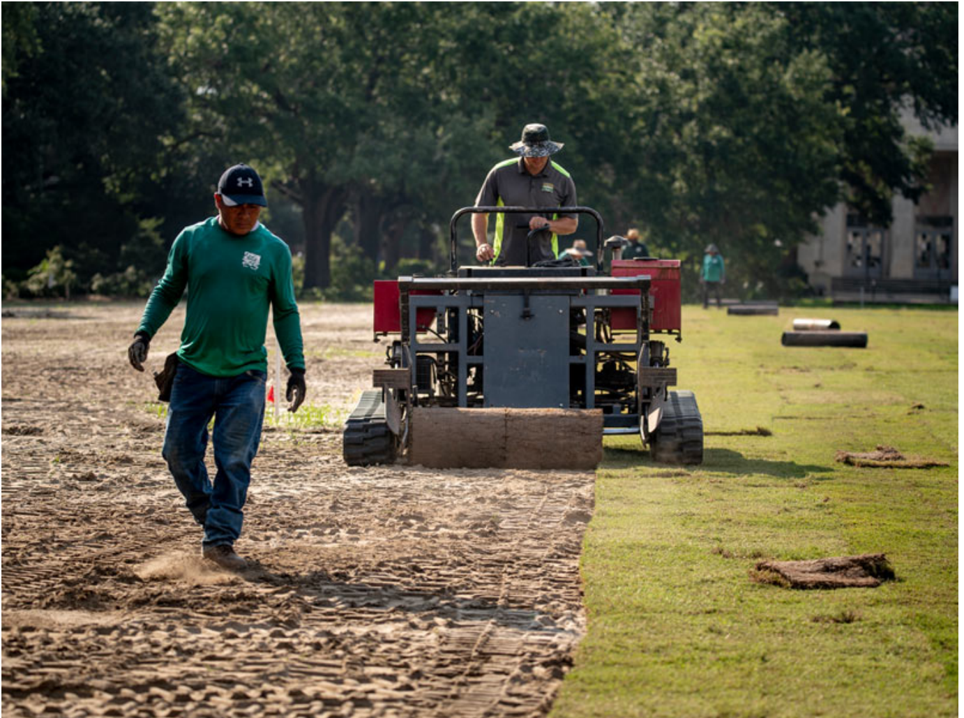
New sod is placed on Berger Family Lawn. The quads on the uptown campus were refurbished after the deconstruction of 13 temporary buildings that included classrooms and a Dining Pavilion. The additional structures were erected to provide more spaces for social distancing within classroom environments. (Photo by Paula Burch-Celentano)
