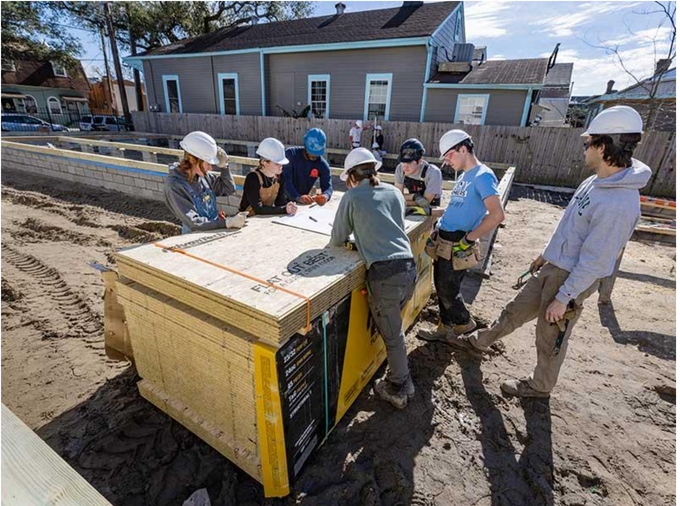
Architecture students Quinn Kelsey, left, Le'Bryant Bell, center, and Ethan Lewis, right, check a floor plank during construction of a home. (Photo by Rusty Costanza) Students go over plans for a home under construction with Sara Allen Harper, front left. (Photo by Rusty Costanza)
