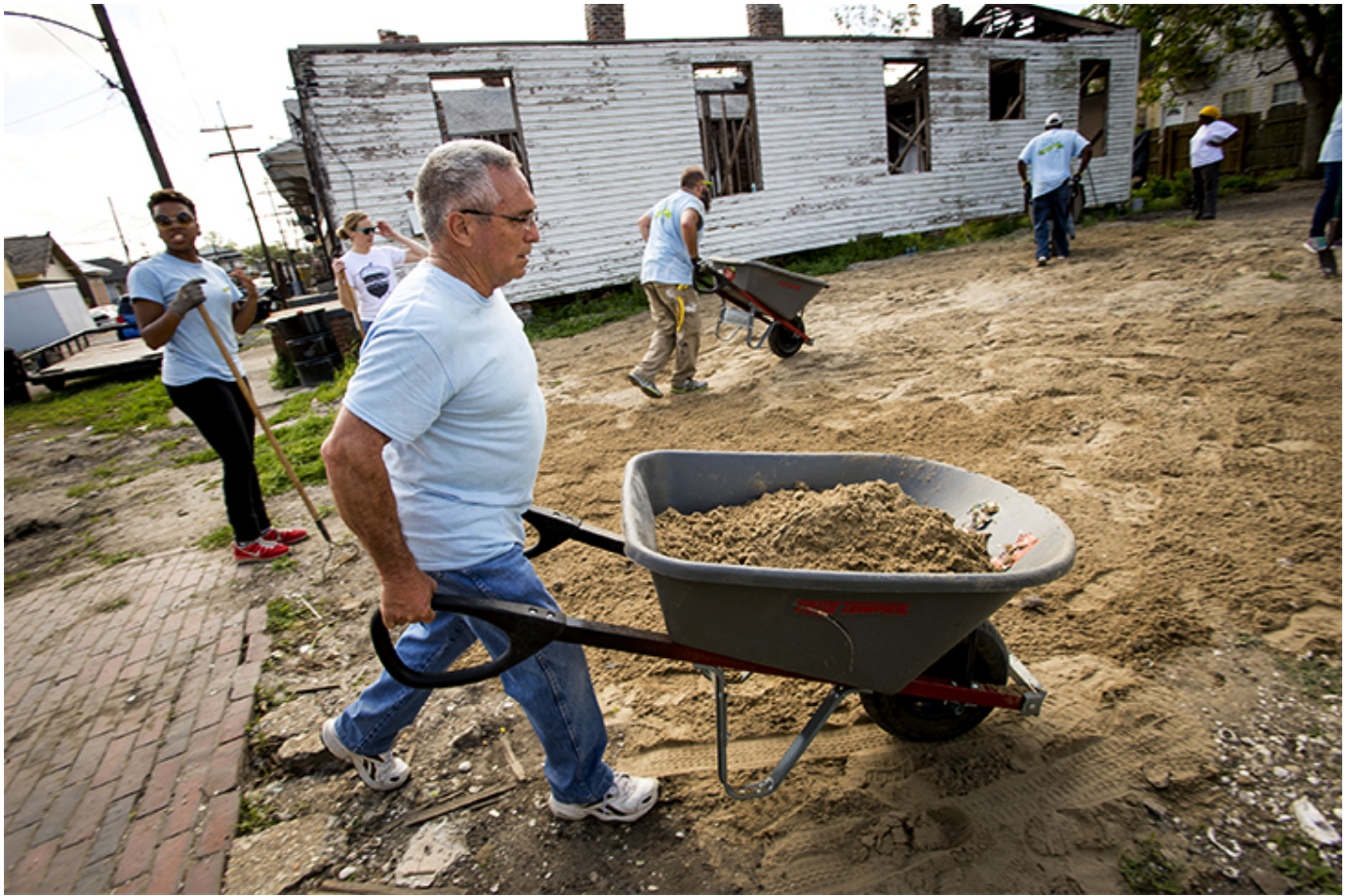
Butsie Duhon, a painter with facilities services, does his part to level a lot in Mid-City.
